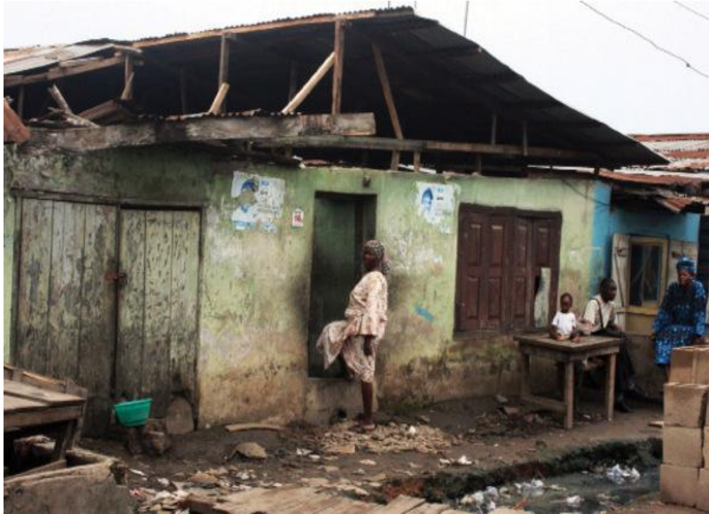
Plate 4.1: Housing condition in Oje, Ibadan
