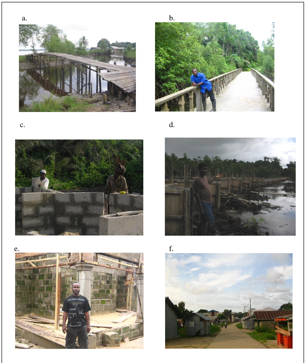
Plate 4.7: Bricklaying and construction works in the study area (a) Local wooden bridge built with mangrove wood connecting Kongho to Kotokiri, (b) Concrete bridge built across the mangrove forests to link Apparanbie community, (c) Bricklayers at work on a building in the study area, (d) Road construction in Minibie community using mangrove wood, (e) Block building under construction in Kotikiri community and (f) View of Sangana community showing access road and buildings
