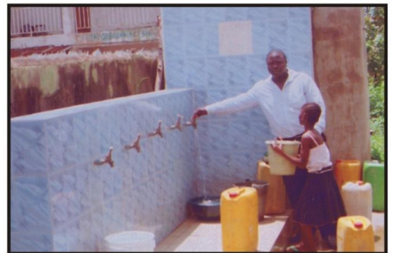
Community Bore Hole at Omupo, Ifelodun L. G. (Plate 8)
