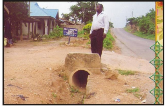
Construction of Culvert by Community Development Association at Country Home, Ede (Plate 34)
