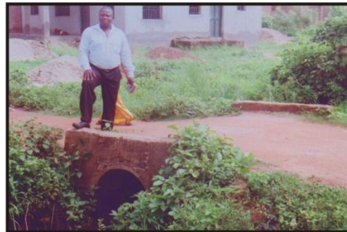
Construction of Culvert and Rehabilitation of Road Galadima Community in Ilorin West L. G. (Plate 32)
