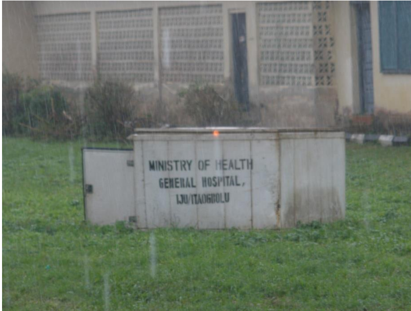
Plate 4.2: Refusedump in the open site at Iju-Itaogbolu Genral Hospital (Akure north LGAs) Source: Authors' feildwork, 2010
