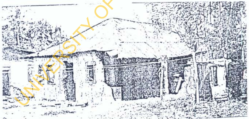
Fig. 26: A mud house in Babamogba Ogundeji village with fallen walls. The room spaces within the fallen walls are used as kitchen pending the time the walls would be rebuilt. The two windows by the left wing of the house are covered with used zinc roofing sheets while the entrance space is yet to have a door frame and covering. (Source: Babajide et al (2006), p. 36)
