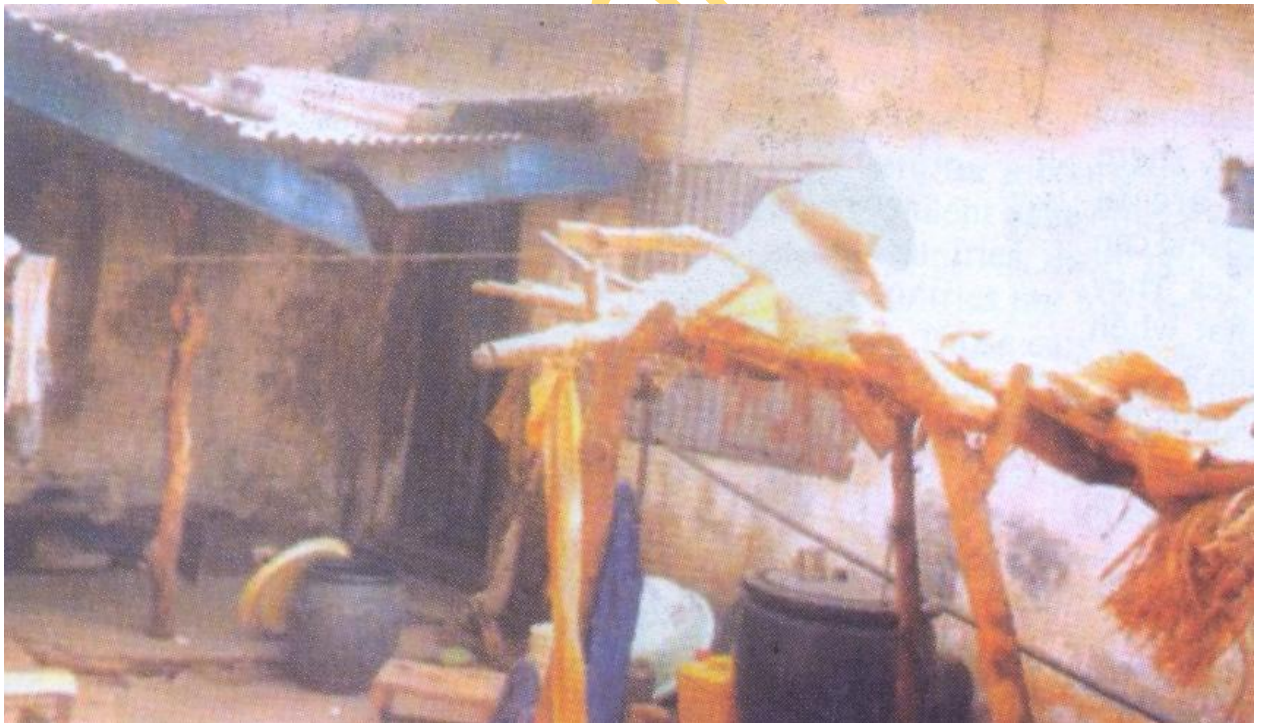
Plate 13: Section of the Wukari Barrack, Taraba State, showing the Present state of destruction in the barracks due to neglect of the welfare of the Nigerian Police Force Source: Field work 2008
