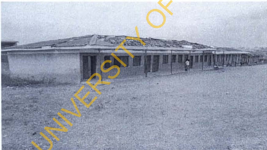
Plate 1: Part of the roof of a building blown off by rainstorm at IMG Primary School, Eleta, in Ibadan Southeast Local Government
