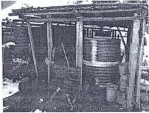
Fig. 11 Failed joint in metal tank, re-soldered and painted over as shown by the white vertical and horizontal strip. Also shown are metal drum and assorted containers which are also used for storage
