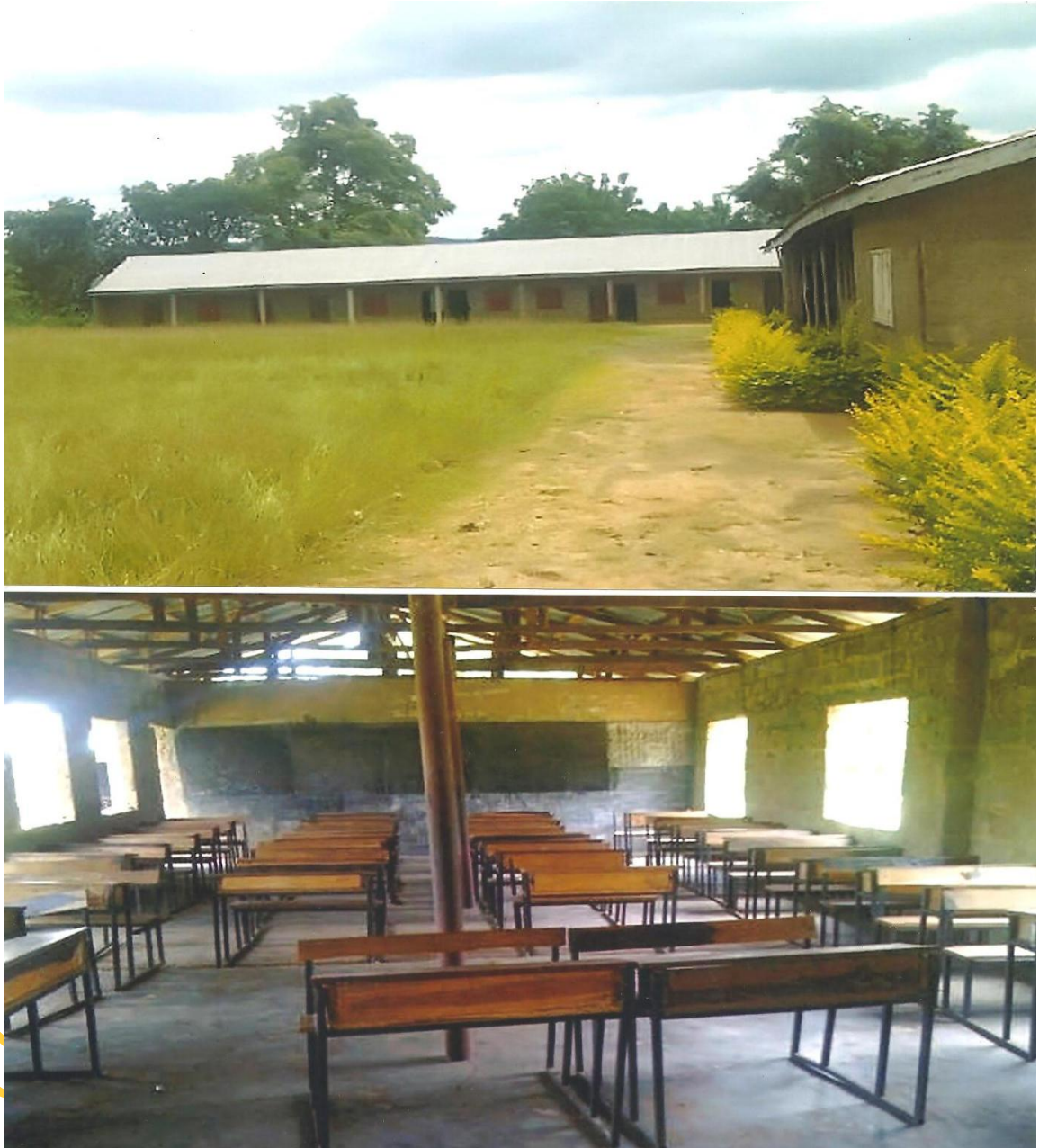
A Block of Classrooms at Community High School (Formerly Christ International Academy), Moriwi, Ogun State.
