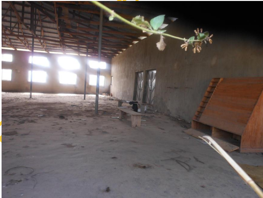
The Internal view of the structure of the Redeemed Christian Fellowship (RCF)
