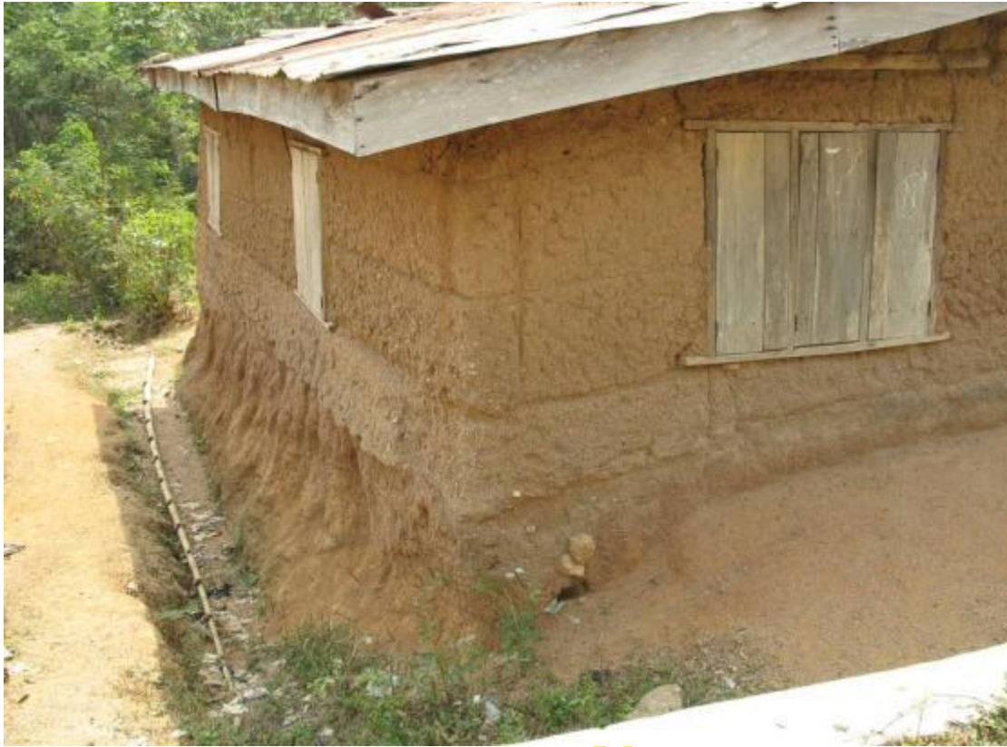
Plate 1.2: Erosion washes at Iresi (Drainage)
