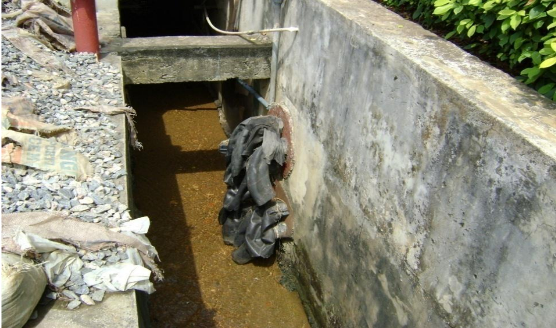
Appendix 6: Effluent channel of Afrab Chem in Isolo Industrial Estate.
