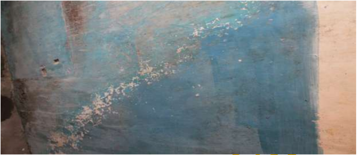
Plate3. 2:Flaking wall paint
