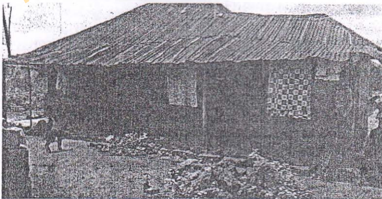
Figure 2: Dilapidated building used as ward for TOSP Patients
