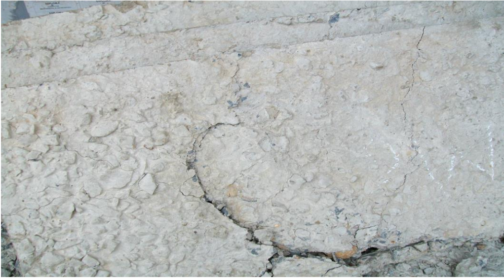
Plate 10: Crack pattern for waffle slab W5 Supported on 1 long side and 2 short sides
