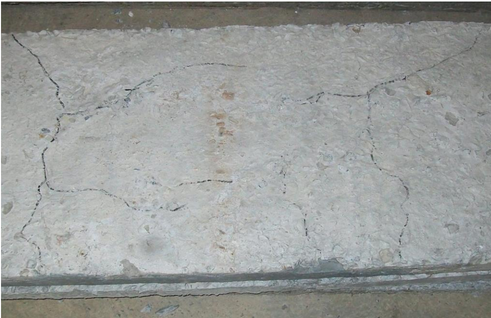
Plate 6: Crack pattern for waffle slab W2 Supported on all 4 sides
