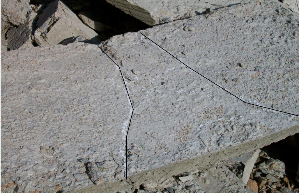
Plate 11: Crack pattern for Solid Slab S5 supported on 1 long side and 2 short sides
