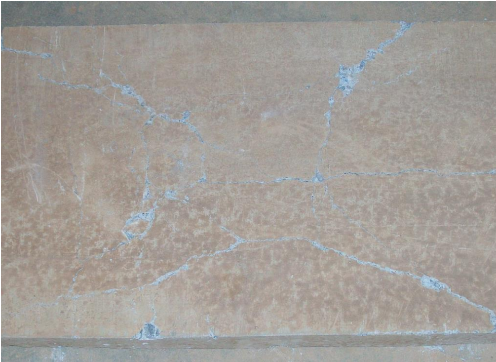
Plate 9: Crack pattern for solid slab S4 supported on all 4 sides
