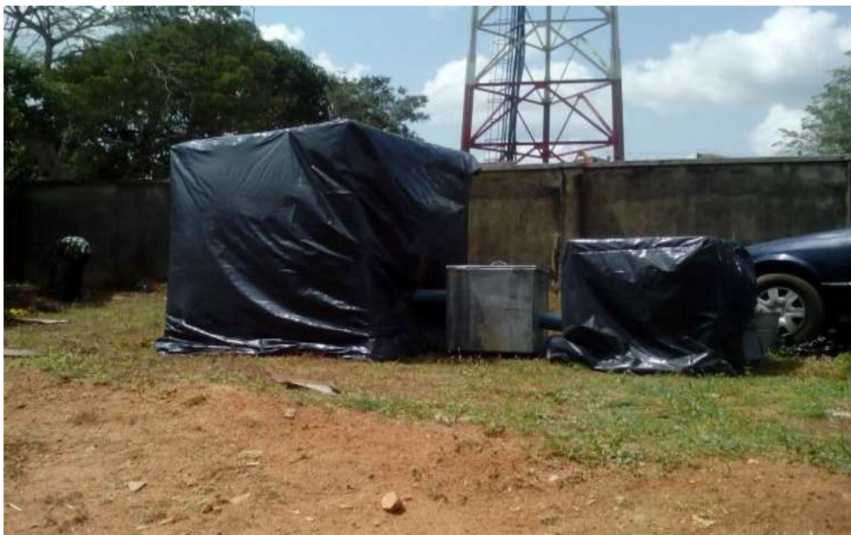
Plate 3.16: Carbon dioxide extractor placed between the covered inlet and outlet chambers
