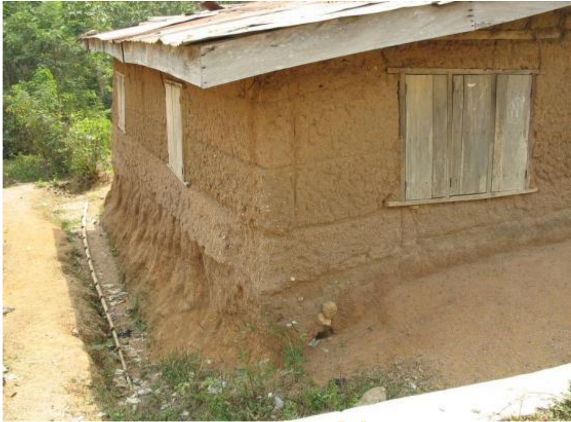
Plate 1.2: Erosion washes at Iresi (Drainage)
